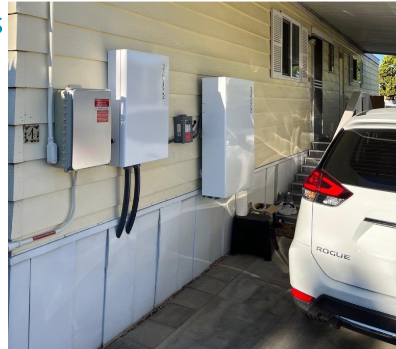
Battery system installed at CEA customer's home at no cost through Battery Bonus Connect.
